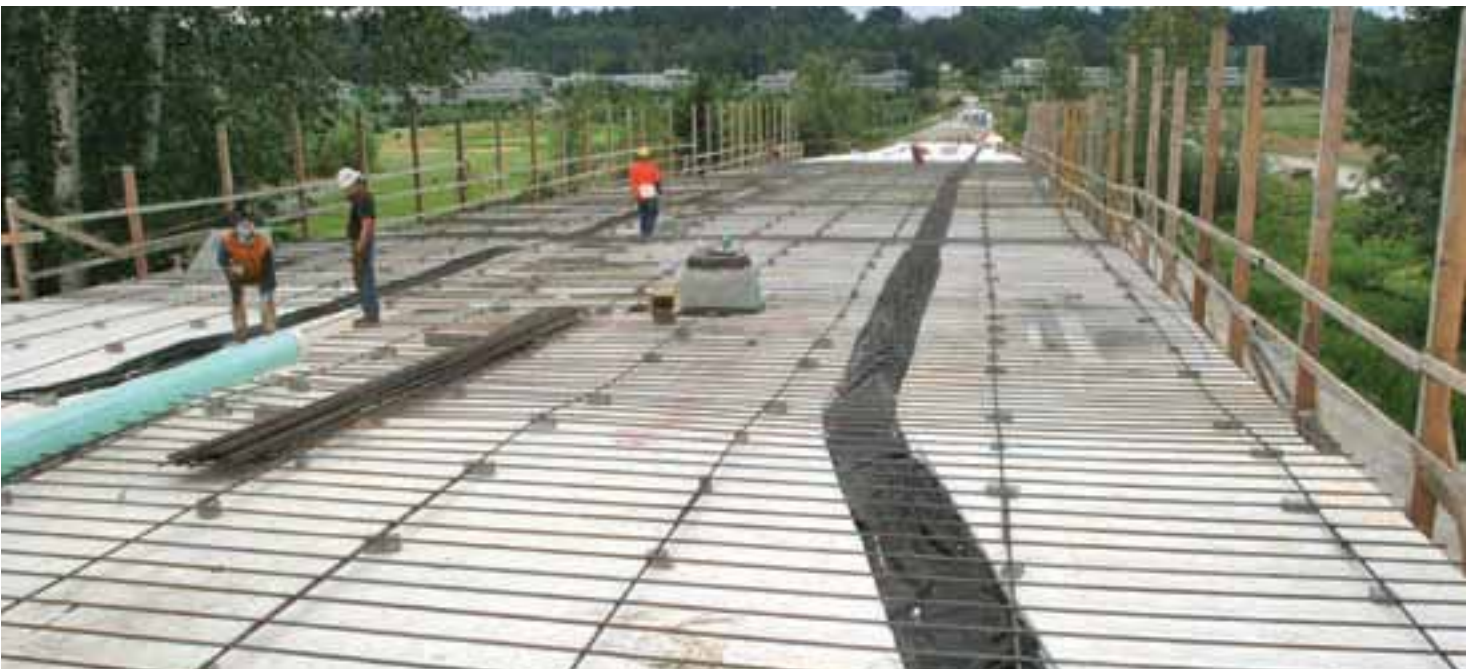
Placement of reinforcing steel for the load distribution slab: The load distribution slab provides protection for the geofoam, distributes live loads and the roadway pavement dead loads, and is used for the top lateral connection for the fascia walls.
