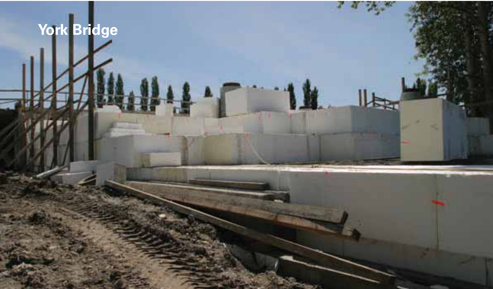
| Embankment getting higher: Temporary timber supports provide fall protection and are not required to hold the geofabric in place.
