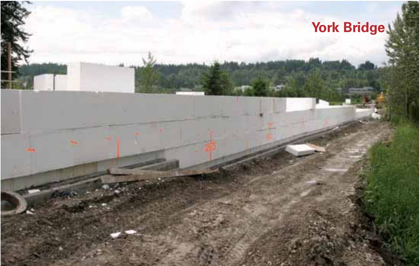
| Embankment continuing to the west: The leveling pad for the precast fascia wall panels is clearly seen in front of the fill.
