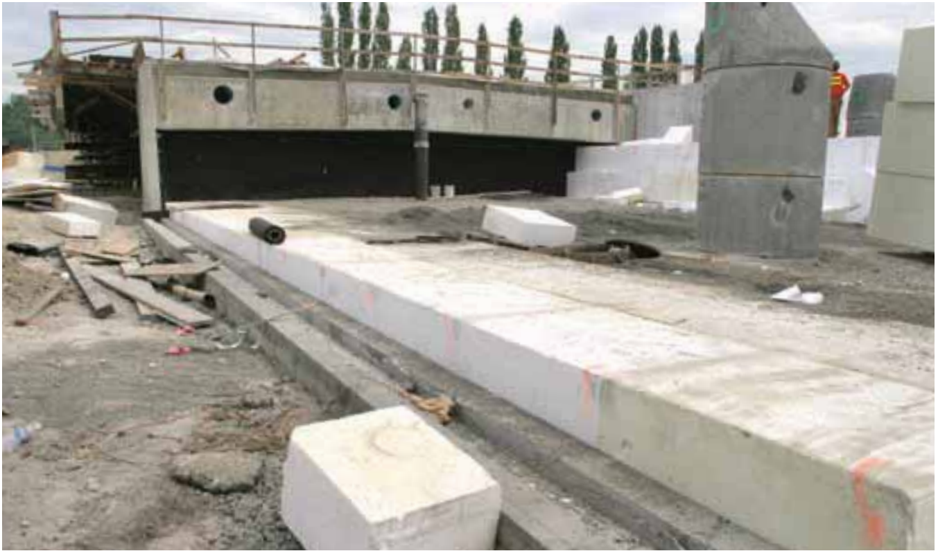
| Geofabric near west York Bridge abutment: Near the west abutment, the geofabric is deeper near the outsides of the fill. This accounts for the added weight of barriers, sidewalks, and fascia panels. On the left is the leveling pad for the full-height concrete fascia panels.
