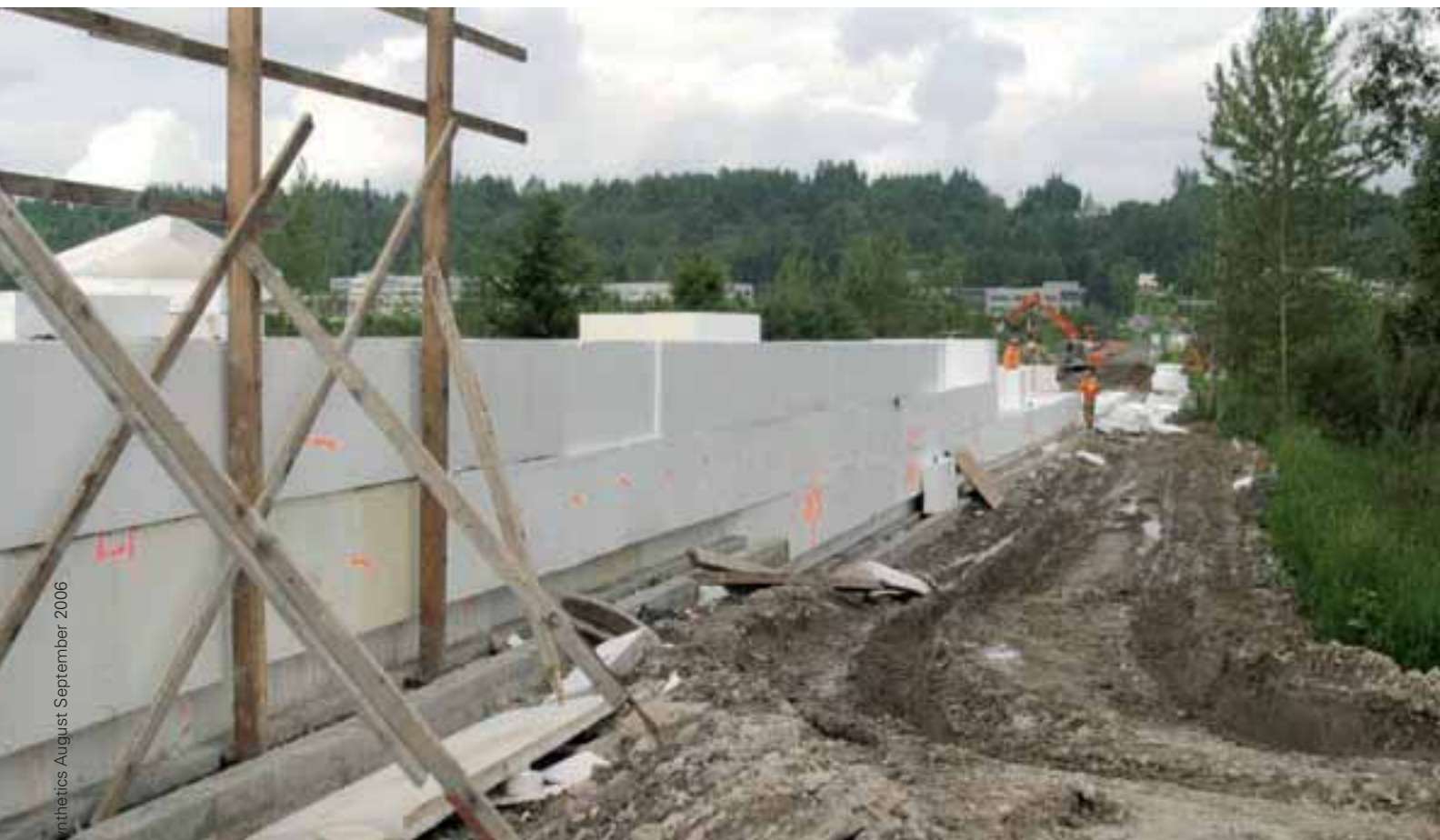
| Embankment looking farther west: The geofabric steps down to follow grade as the fill is placed from east to west.
