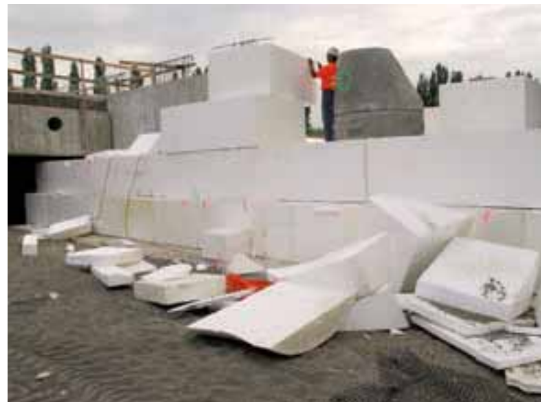
| Geofabric cut around utilities: Blocks of geofabric sit on a sand drainage and leveling blanket. The sand layer is placed above geotextile reinforcement, over existing ground. The geofabric is cut to fit around the utilities.
